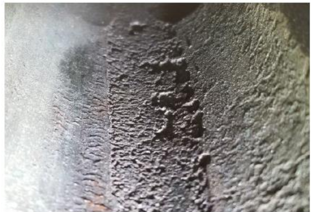
Jt #258: Pitting in wear
