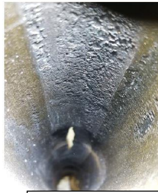
Untreated Joint 292 failed due to sucker rod wear that thinned the wall
